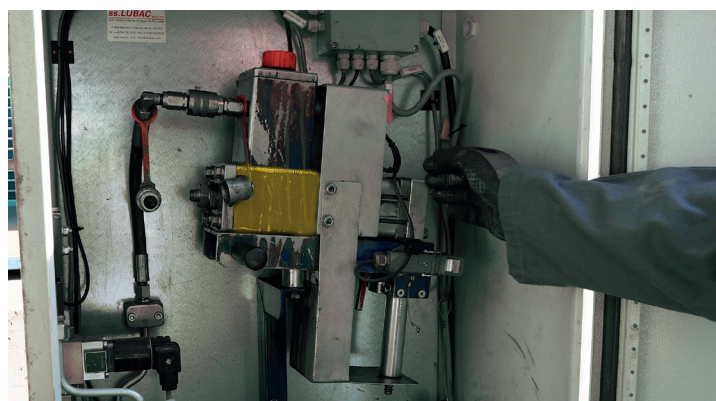
Safely stowed away: filling station including automatic filling device of the ss. LUBAC Ring Star at the LEUBE cement plant
