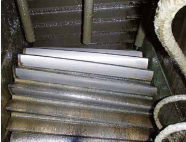
Figure 4: Pinion / girth gear with Klüberfluid C-F 3 Ultra: inspection and documentation made easy with strobe light or high-resolution digital camera while running.
