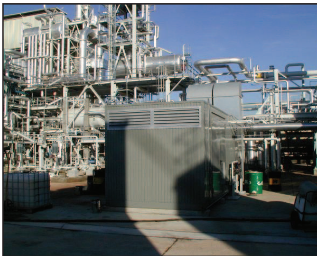
■ Rotary screw compressor in a sound proof housing in a refinery.
