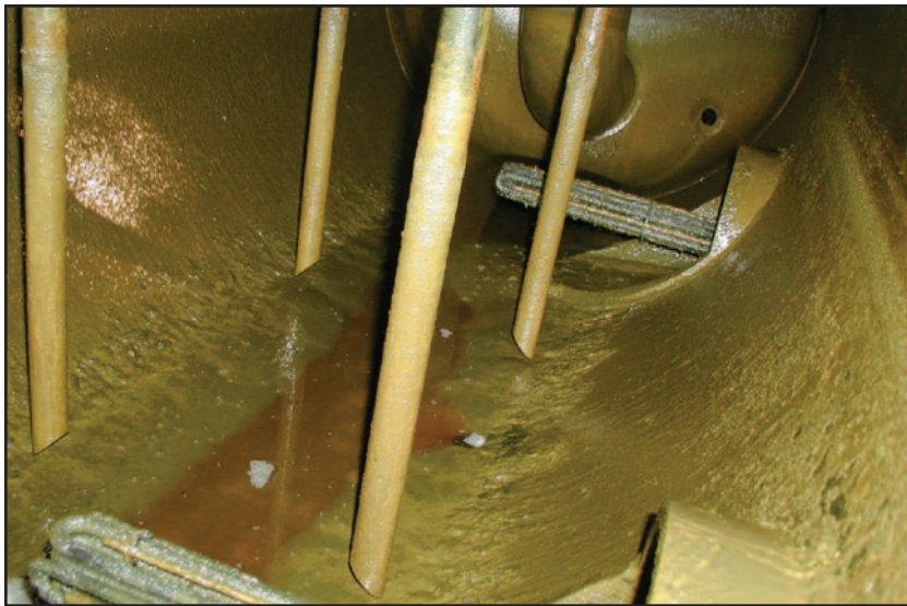
■ Oil container of a process gas compressor, covered with greenish sludge from reactions between the lubricating oil and the process gas.
