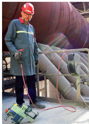
Compressed air supply at ring #2
